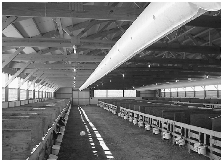
Fig. 5. A positive-pressure distribution duct installed in a naturally ventilated calf barn. The fan that powers the system is installed in an outside wall and forces air into the tube. Holes are punched at 4 o'clock and 8 o'clock positions in this barn and sized so that air exits the holes at about 800 ft/min. The small volumes of air are driven into the pens between the solid panels. In this barn, the airborne bacterial counts in the pens dropped from 170,000 cfu/m 3 to approximately 40,000 cfu/m 3 and the annual number of calves treated for respiratory disease was reduced by approximately 75% following the installation of the supplemental system.
